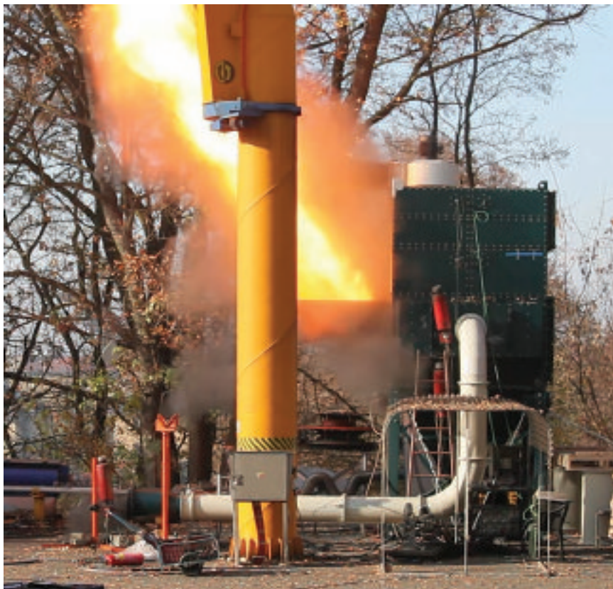
Figure 3: Almost immediately, the flame is extended away from the dust collector and into a safe area. Courtesy: Camfil Farr APC
